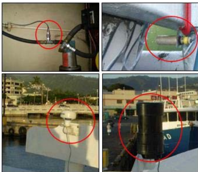
Figure 4. Examples of sensor installations on the project vessels: hydraulic pressure sensor (top left), drum rotation sensor (top right), GPS receiver (bottom left) and satellite modem (bottom right).
