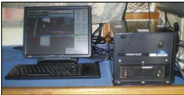
Figure 5. Example of monitor, keyboard, and EM control box installation in vessel wheelhouse
